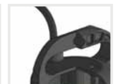
Power cable export insulation treatment. No water leaking.
